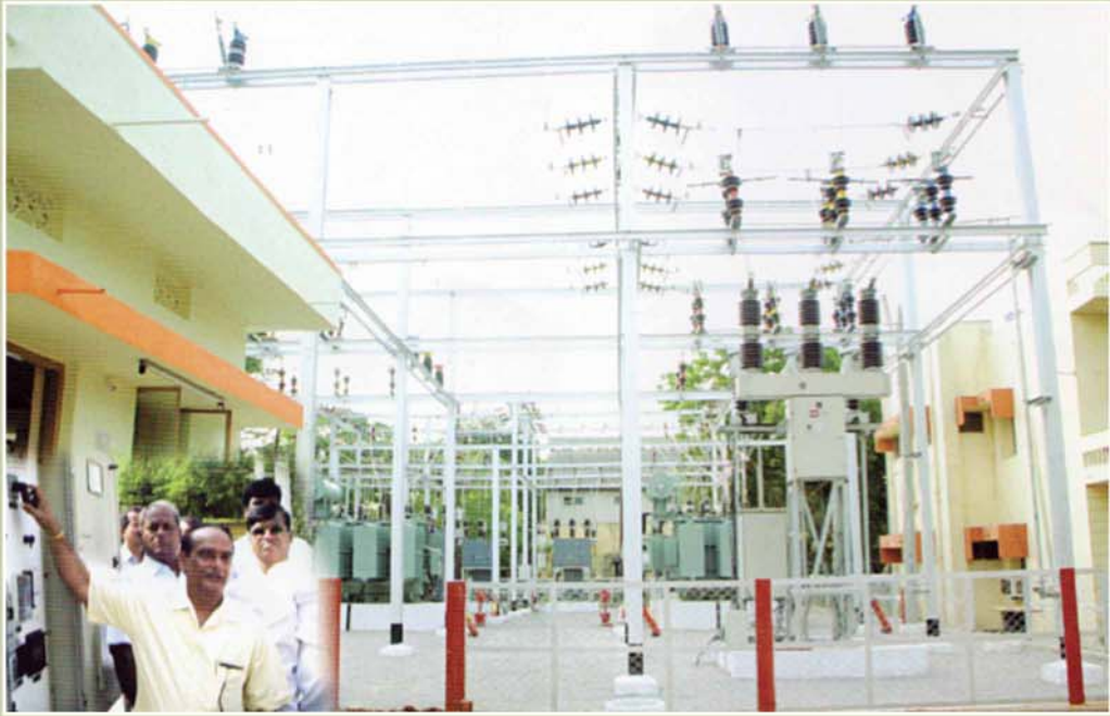
Inauguration of New 33/11 KV Sub-Station at Nakkalagutta, Hanamkonda. on 28 th October 2009 by Sri Ch. Narasimha Reddy CMD, APNPDCL
